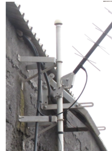
Comms & Power System
