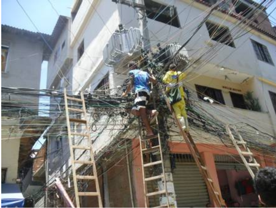
Figure 1.2: Example of power distribution infrastructure manipulation a .
