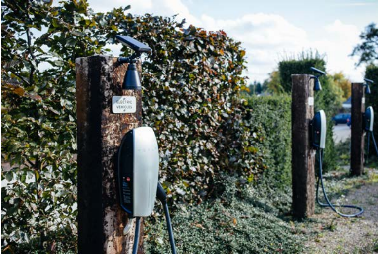
Figure 7.17. Electric vehicles chargers attached on wooden posts. Source: author's own photograph.
