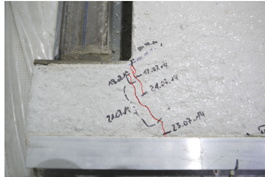
Figure 3.37: Corner 2 with cracking path
