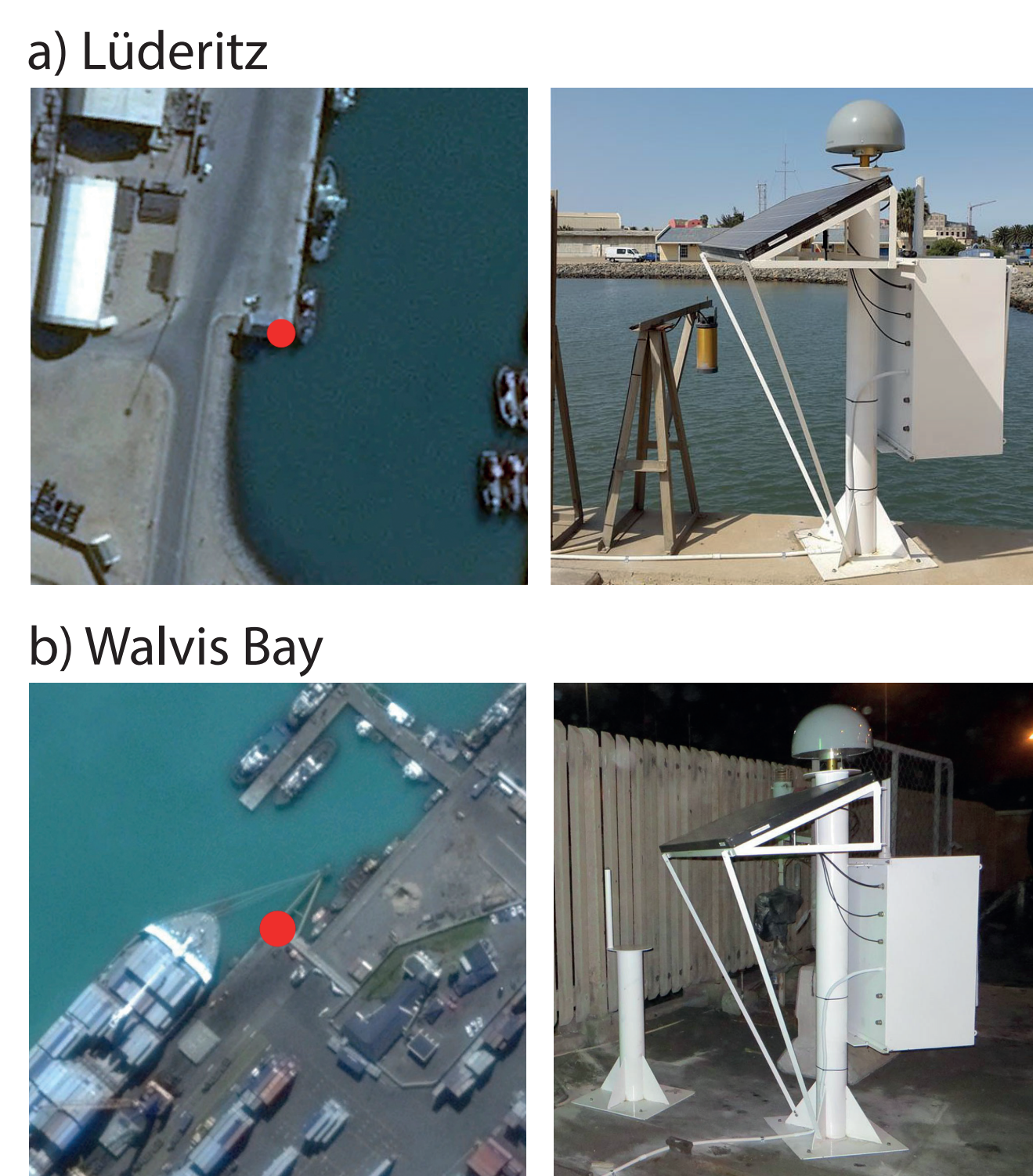
Figure 2: New continuous GNSS @ tide gauge stations in Lüderitz (a) and Walvis Bay (b). Marine-grade stainless steel monument and enclosure with electronics and auxiliary equipment.
